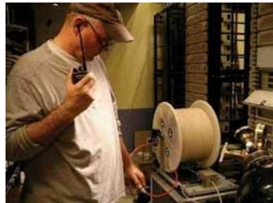
An installer from Ascent Media Systems & Technology Services prepares to blow fiber into a section of the Time Warner Center.
