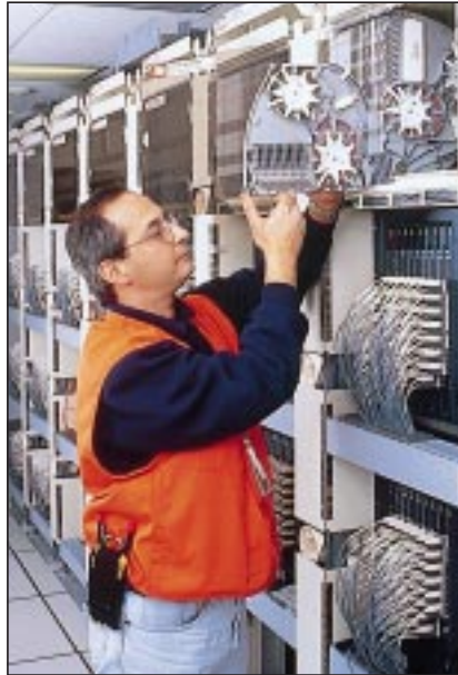
During an air-blown optical-fiber installation at the Getty Center in Los Angeles, technician Vasken Bezjian of AIDCO Inc. (Chino, CA) inserts a splice-holding connector card into the FibrMax 2700 fiber management system from 3M Telecom Systems Div.
