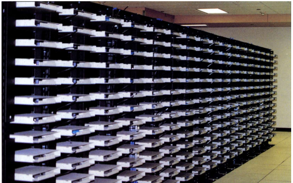
In the telecommunications closet are rows of fiber distribution panels and patch panels in data management racks.
