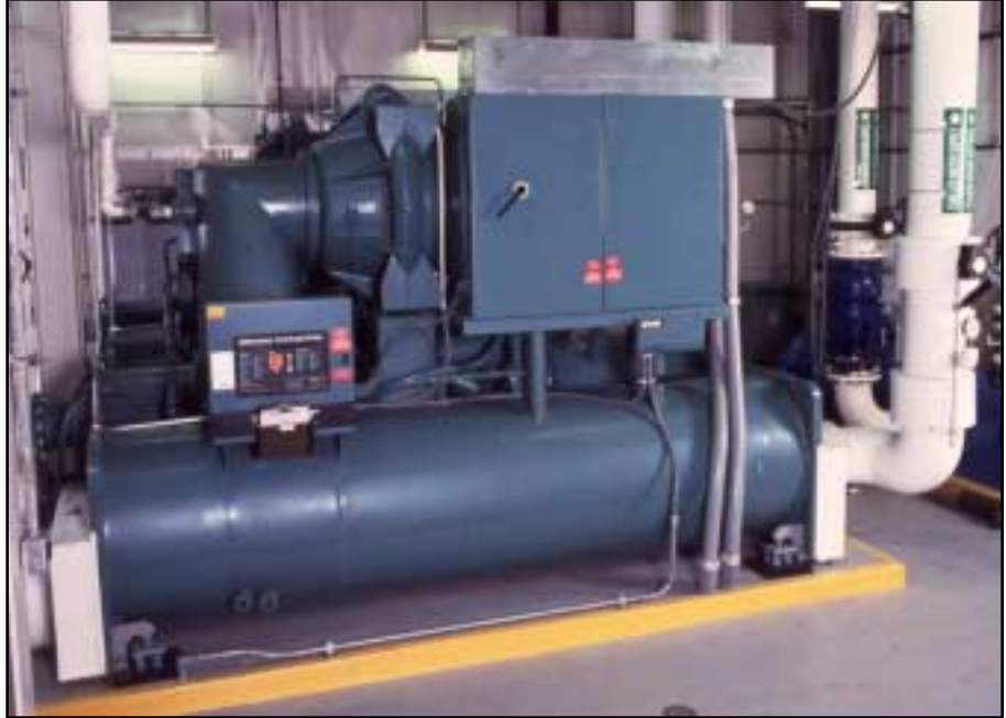
In a phased renovation plan, the NPS designed and engineered a centralized chilled water plant and FutureFLEX ABF data communications network for automated control of its HVAC and other systems.
